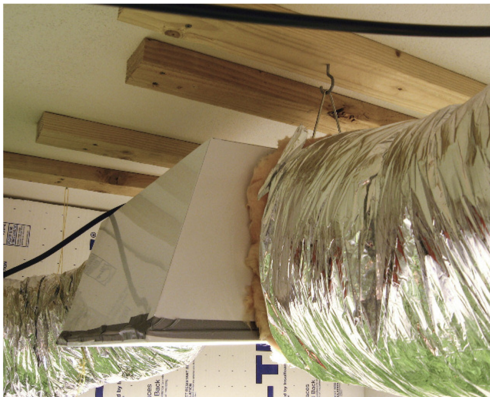
Insulated ducting on the air-cooled lights.
