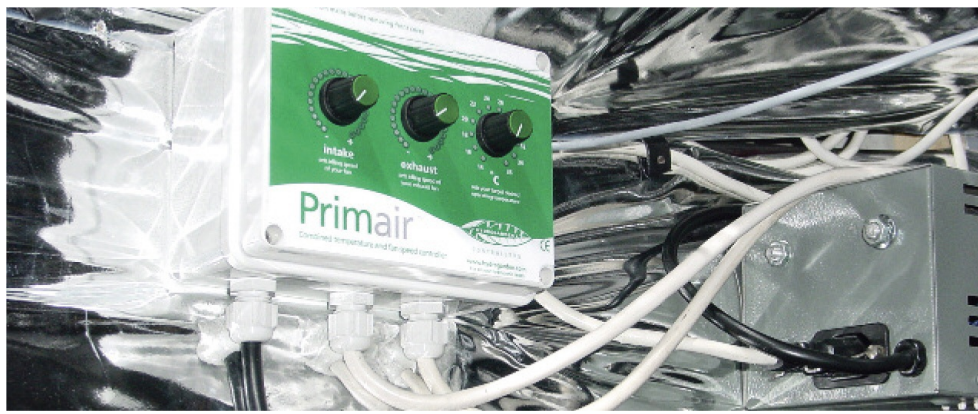
Air intake, exhaust, and temperature controllerX.
