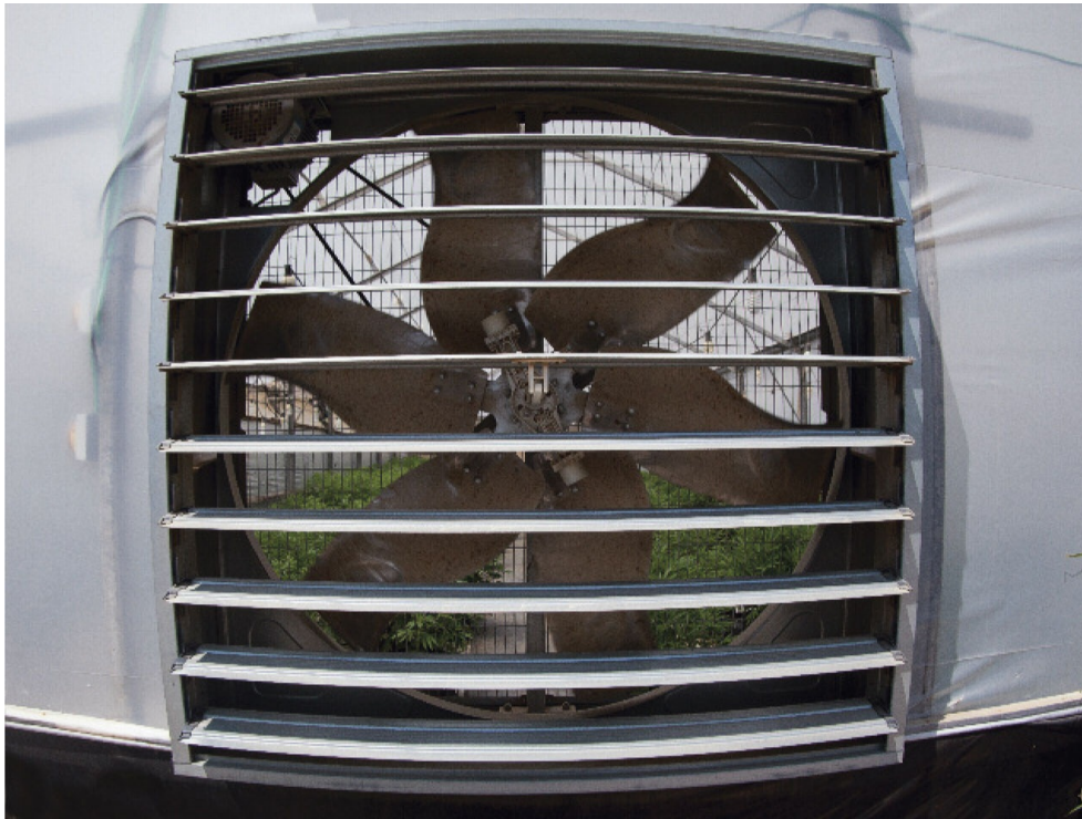
Extraction fan to keep humidity and temperature levels appropriate in the greenhouse.
