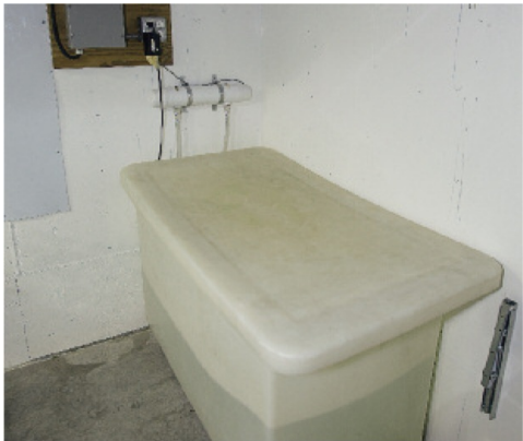
Lid on the reservoir for cleanliness and to minimize humidity by limiting water evaporation.
