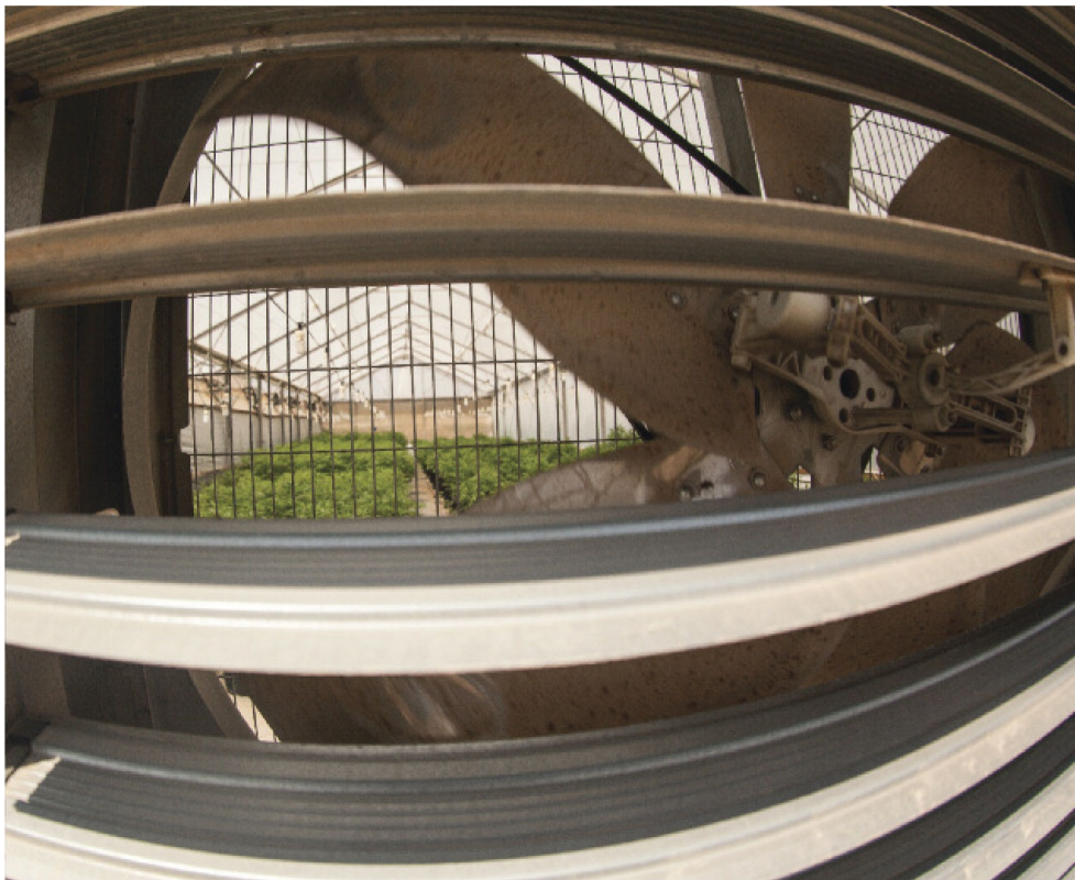
Greenhouse extraction fan seen from exterior of garden.
