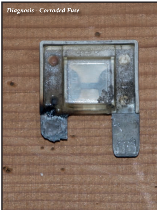
Diagnosis - Fuse Housing with remains of the spade leg
