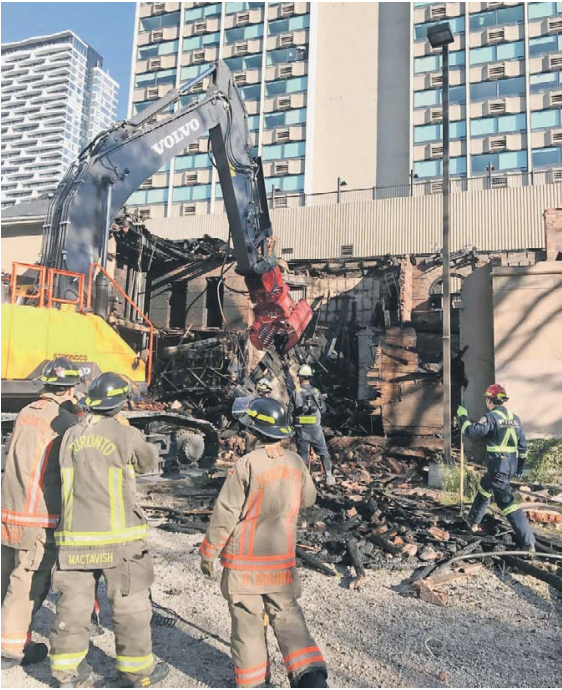
Firefighters had to remove the house’s south wall after the fire, and its west wall was deemed too weak afterward. GRAYWOOD DEVELOPMENTS
