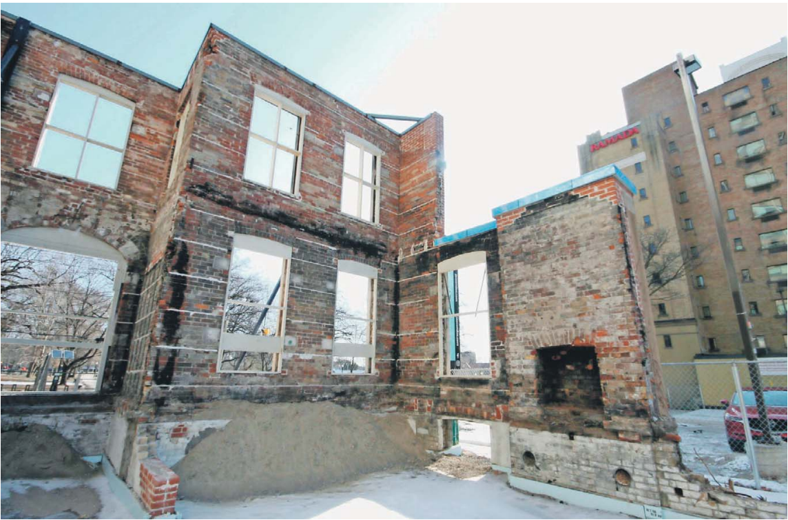
Only the north and east walls are still standing at 314 Jarvis St. after the second fire. DAVE LeBLANC/THE GLOBE AND MAIL
