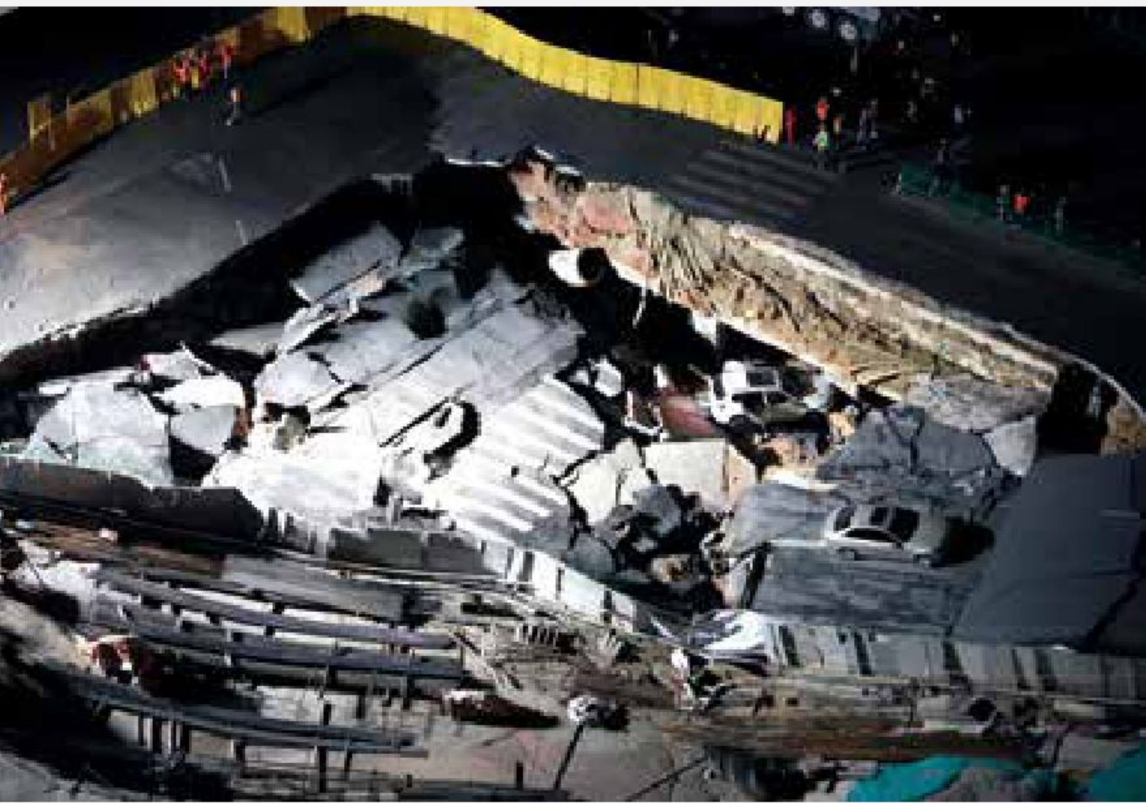
Two cars fell into a sinkhole that opened up at a subway construction site in Xiamen, Fujian Province, December 12, 2019. The occupants were rescued
