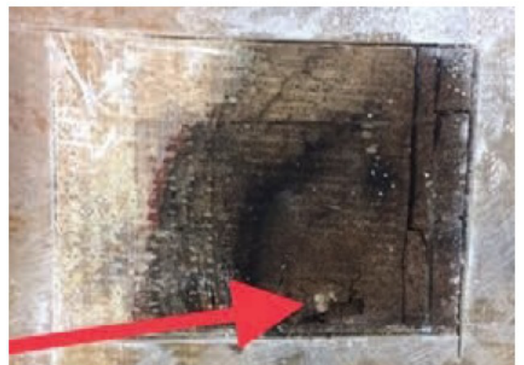
You can see, with the skin removed on the underside of the hatch, the darker, more rotted wood around the column of epoxy putty.
