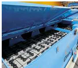
The lead acid battery cells: There is a similar compartment on the other side of the loco. BOTH: CHRIS MILNER
